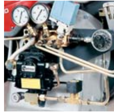
Example of the hydraulic circuit on RL70/M burners
